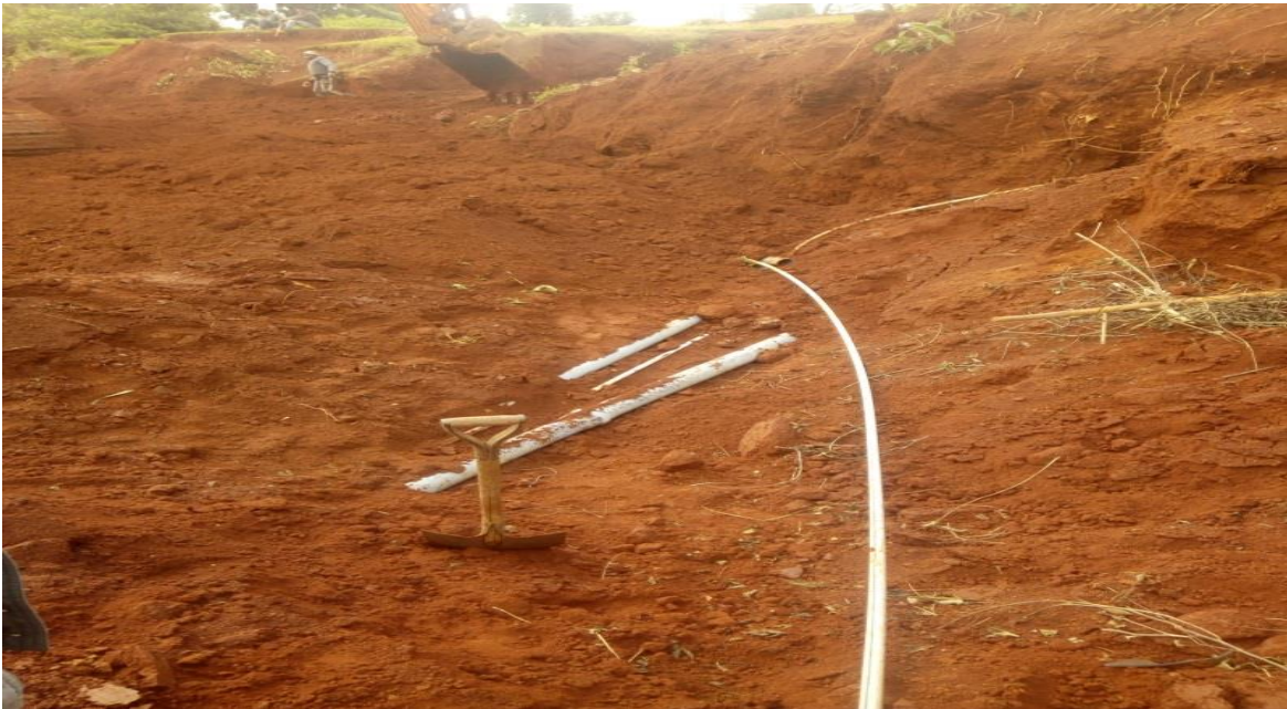
Pipe Damage During Road Construction
